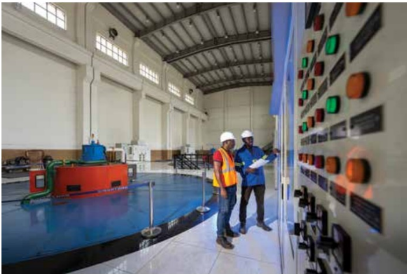
↑ Grand Poubara Hydro Electric Scheme has 200 MW of installed capacity
