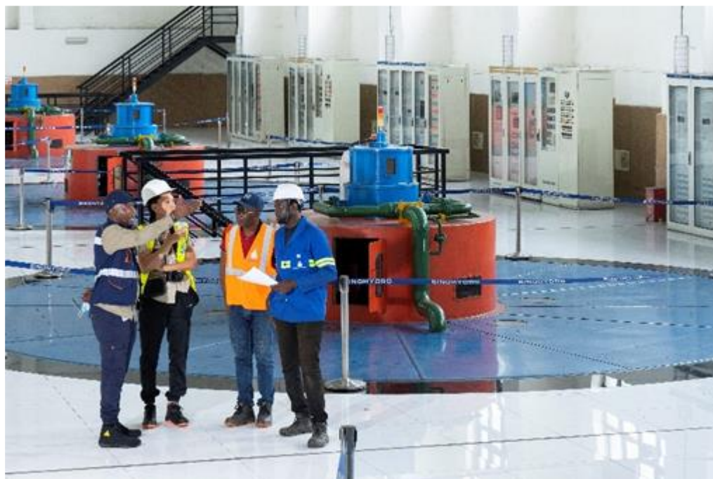
Figure 10: Grand Poubara Hydroelectric Station
